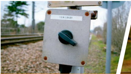
Example of a TOWS switch
