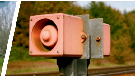
Example of a TOWS warning siren
