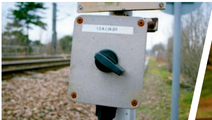
Example of a TOWS switch
