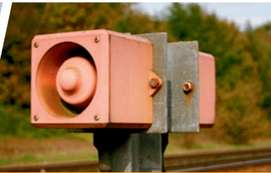
Example of a TOWS warning siren
